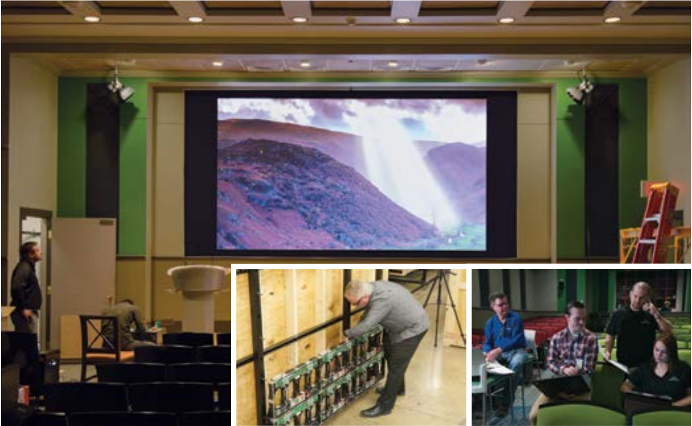
Video wall installation, Humana, Louisville, KY INSERTS: Set-up and testing at Draper, employees working with installers on-site.
