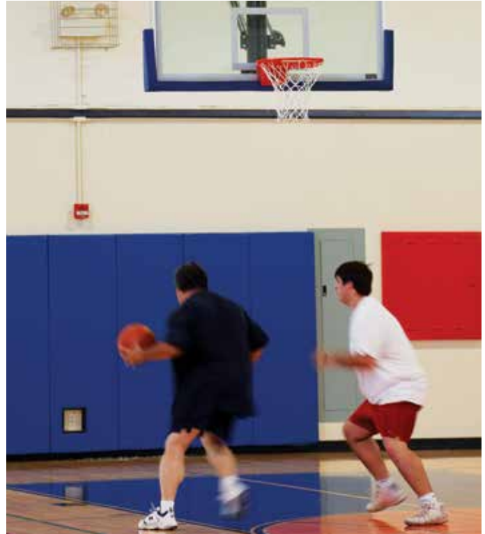
An example of improper padding—there is too much unpadded wall.
