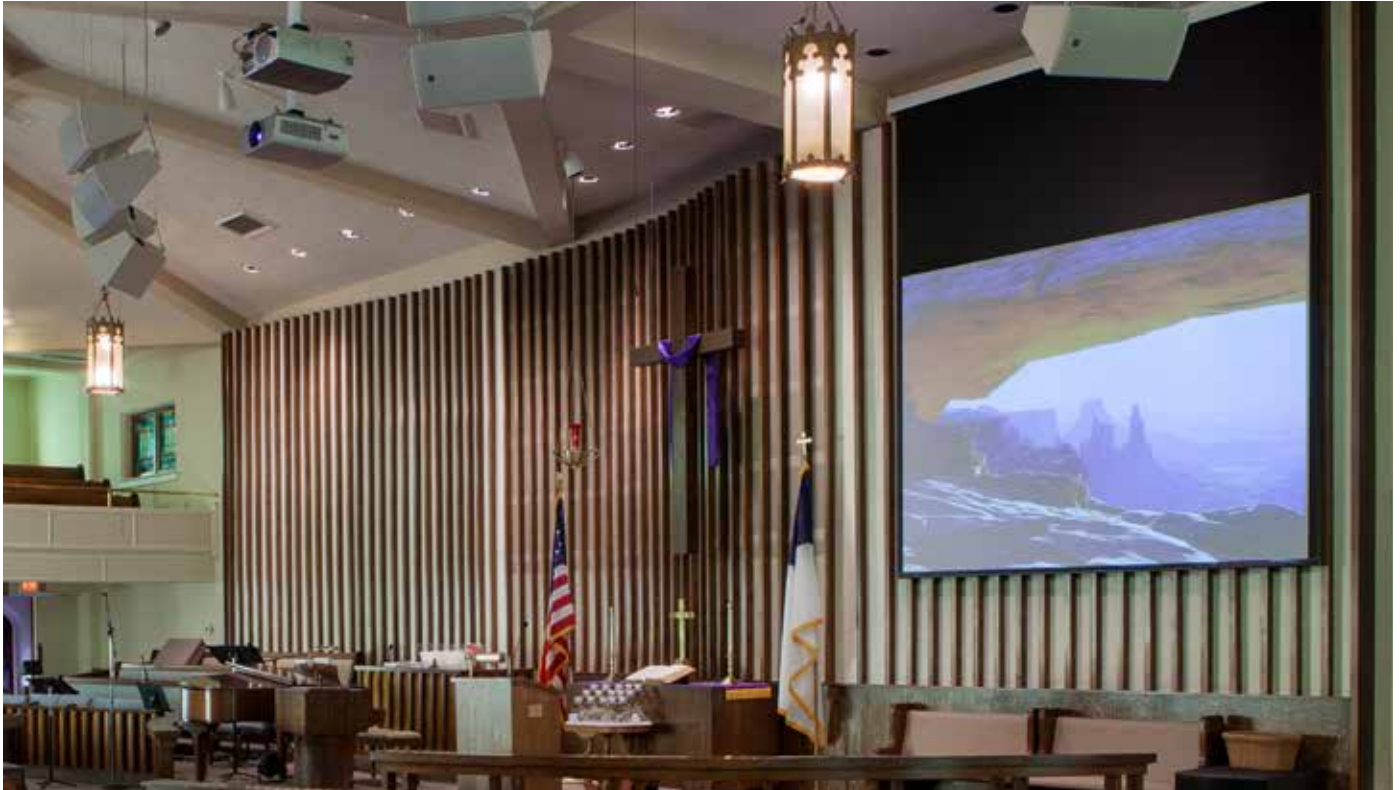
Product: Targa (above) and Edgeless Clarion (lower left) projection screens Installation: First United Methodist Church in New Castle, Indiana.
