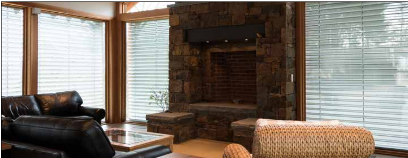
The Omega Blinds provide precise solar control, in addition to privacy. The blinds tied into the lighting controls via dry contacts.
