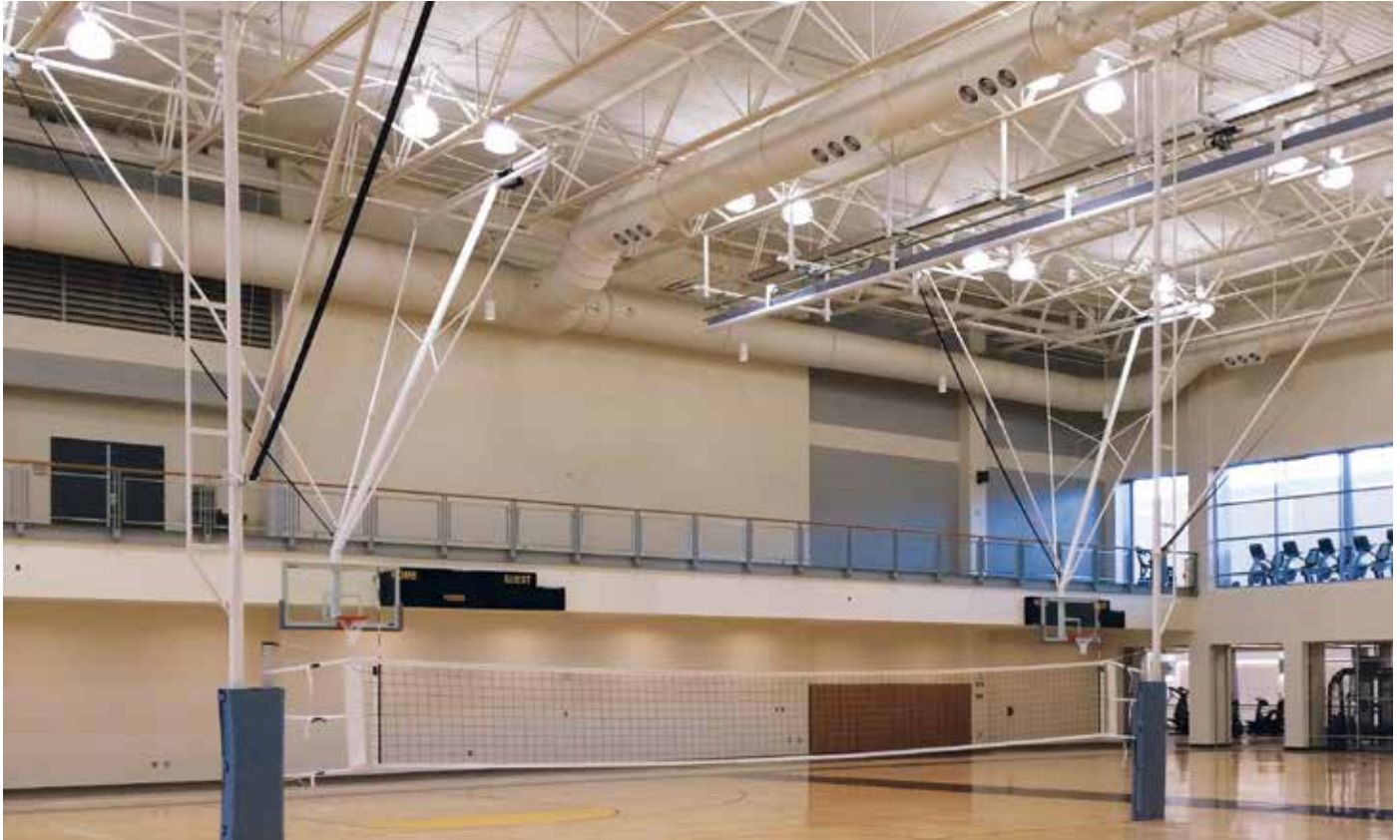
Draper custom backstops and Overhead Volleyball System, part of an installation in the Kennesaw State University Student Recreation Center.
