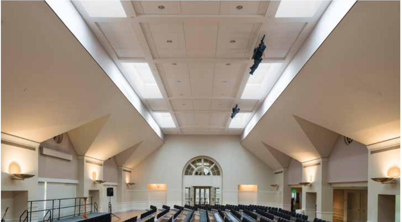
FlexLouver Rack Arm System installed at First Presbyterian Church, Houston, Texas. Photos by Barry Champagne, Houston, Texas.
