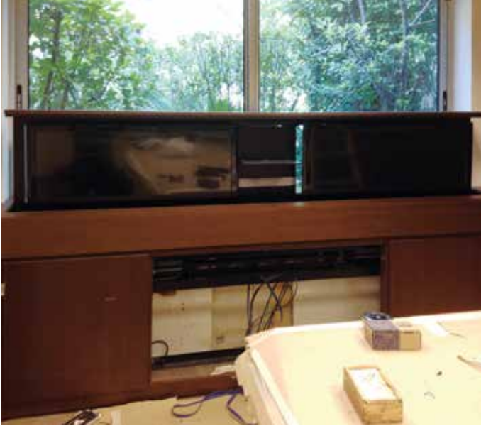
Pictured during install. Control Central convinced Banco do Brasil that the monitors should be out of the way when not in use, allowing the nice view from the windows to be enjoyed when no videoconferencing is taking place.
