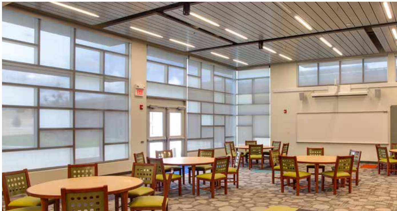
Motorized Shades using Sun Solutions Controls., Alcalde Elementary School, Espanola, NM., Architect: FBT Architects., Photography: Matt Oberer, Matt O Photo Albuquerque, NM.
