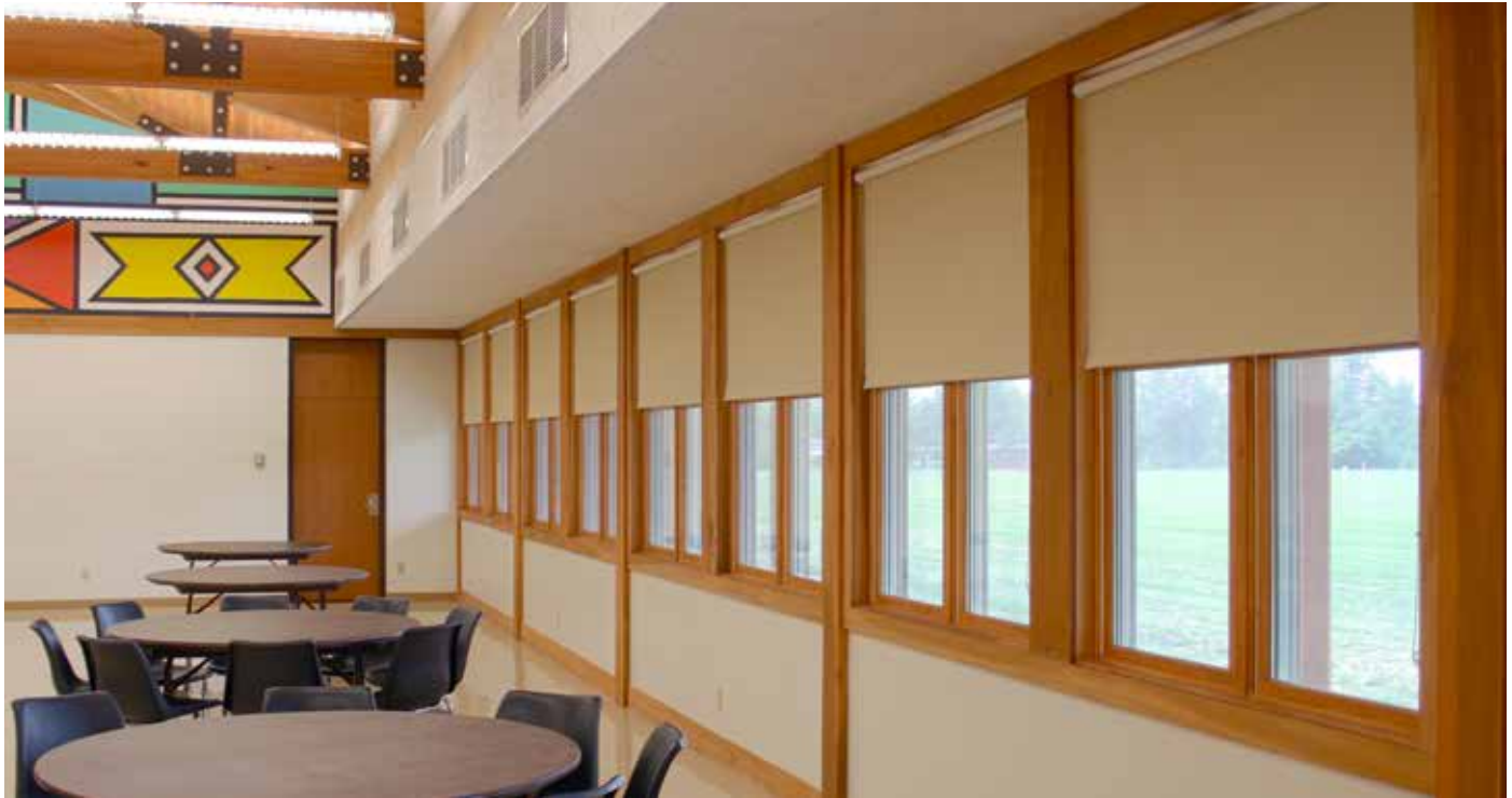
Techmatic Roller Shades, Earlham College, Richmond, IN., Photography Draper
