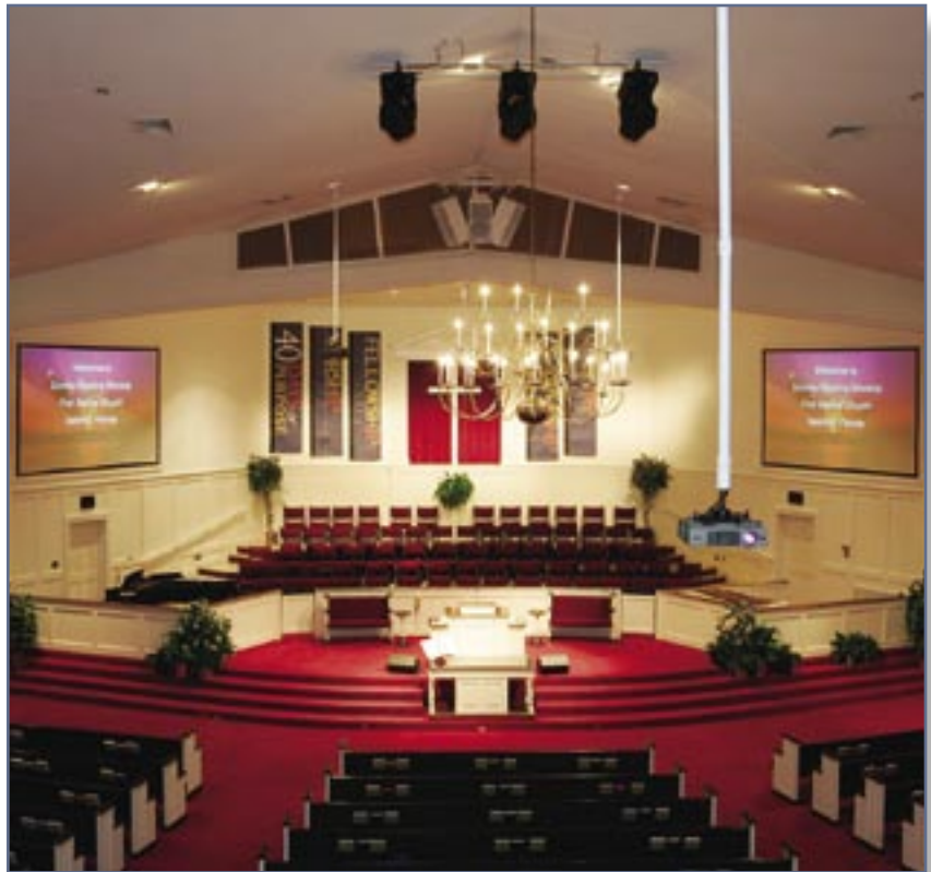
Three Accuset mounts field painted white. The two seen in the background hold projectors that display onto the Cineperms flanking the front of the sanctuary. The projector on the mount in the foreground is projecting onto a Clarion located on the back wall for members of the choir and pulpit staff. Location: First Baptist Church of Sebring, Florida. Design/Installation: Bassett Electronics, Inc., Sebring. Photography: © 2005 Kent Smith, Charlotte, NC.
