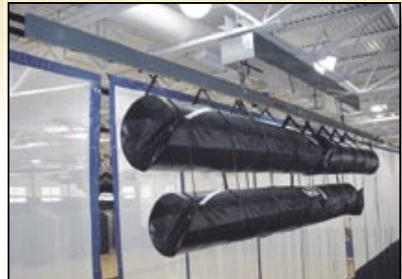
Stationary Double Mat Lifter at Evans Brandt Central Schools, Angola, NY. Architect: Mach Architecture, Buffalo, NY. Photography © Michael Ciurzynski, Lancaster, NY.
