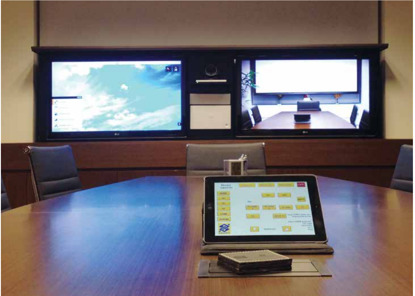
Draper's custom motorized lift solution brings dual monitors up for videoconferencing in Banco do Brasil's Santiago, Chile offices. Installation by Control Central, Santiago, Chile. Photos by Juan Carlos Herrera.
